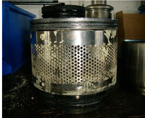
Sulphur deposits in subsurface valve
