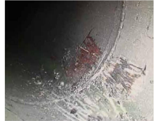
Pipeline corrosion by sulphur deposits
